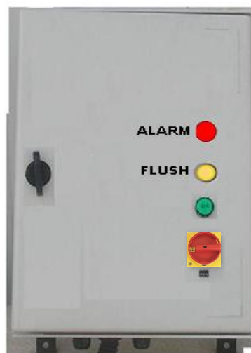
Control unit ELI-02/PLC
